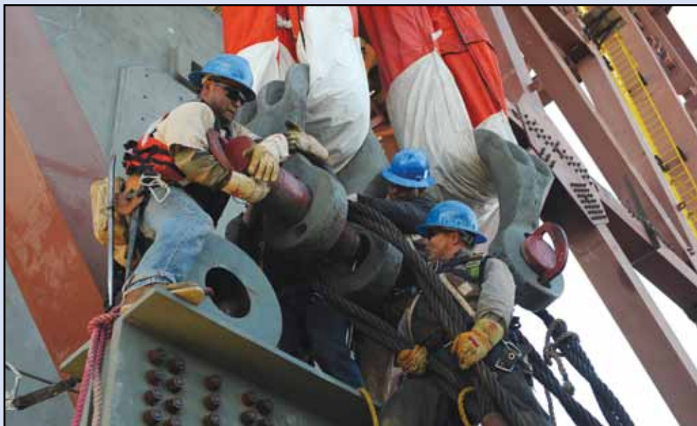
Ironworker foreman Carlos Valverde and Ironworkers Josh Galvin and Augie Solis work hard to take a cable off a shackle, 2010.
