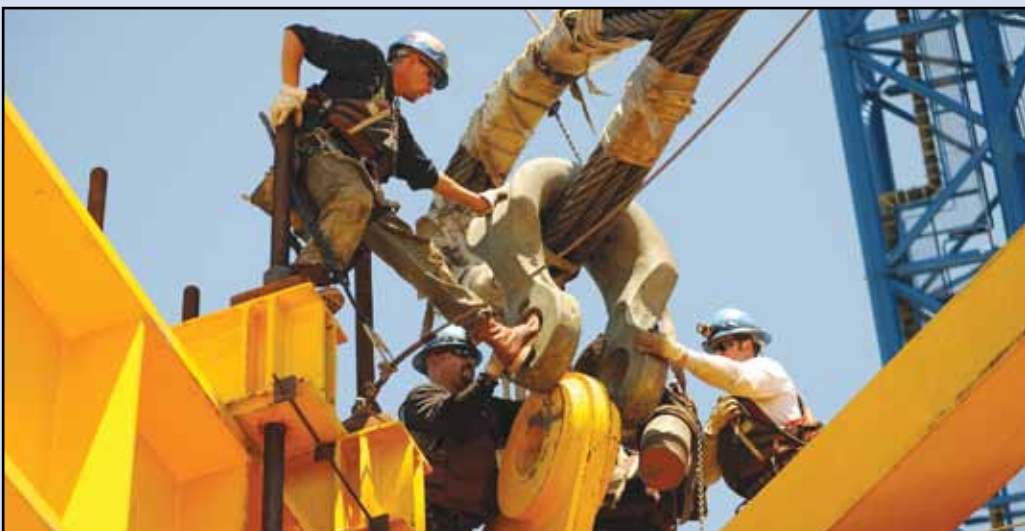
Ironworkers C. J. Biskner, Matt Cochran and Jerry Kubala connecting 600-ton shackles and heavy rigging to OBG deck lifting frame lug, 2010.
